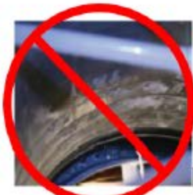
Improperly adjusted TXV
