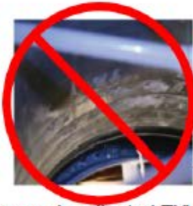
Improperly adjusted TXV
